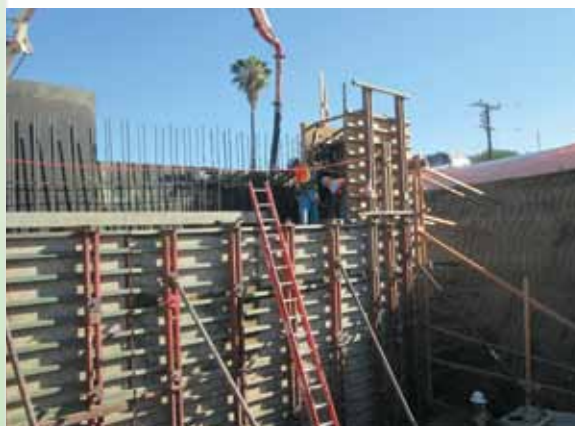
Crews place forms and prepare to pour concrete at the D Street bridge in Perris.
